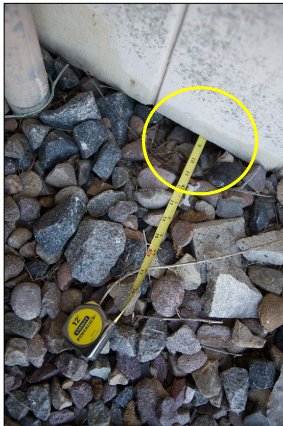
Figure 4-11. Maintain facilities infrastructure, eliminate rodent entry-points (such as holes), and make building repairs quickly to discourage rodent harborage.
