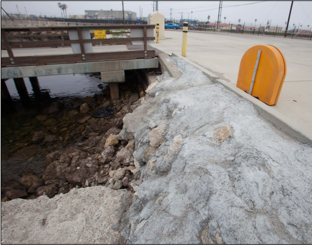
Figure 3-16. NBVC Port Hueneme currently manages potential rodent harborage by pouring concrete into holes to dissuade animal usage.
