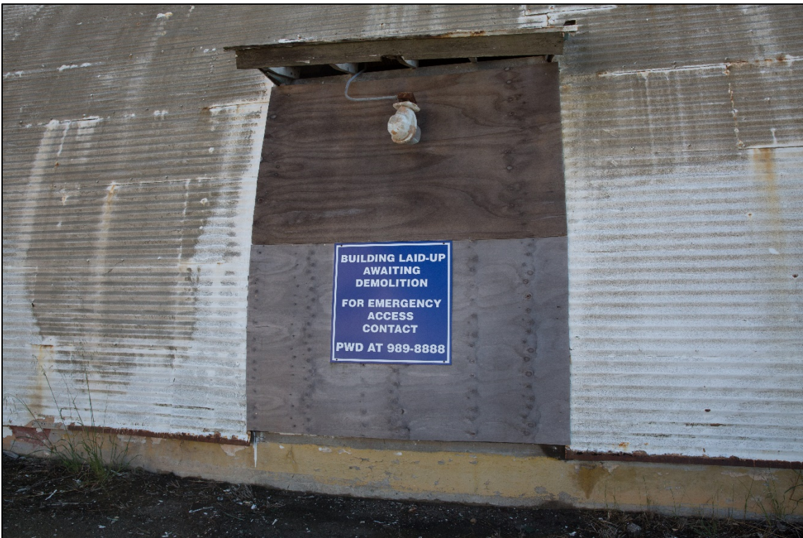
Figure 4-6. Buildings laid up for demolition should be prioritized for quick demolition to eliminate refuge for mesopredators and other invasive species.
